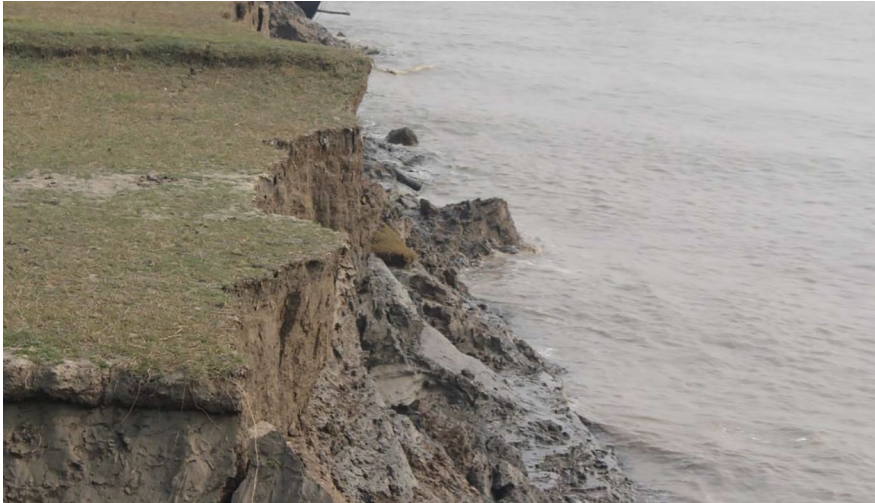
Fig. 4 Unprotected coastal boundary land (Source: Field survey, 2019)
