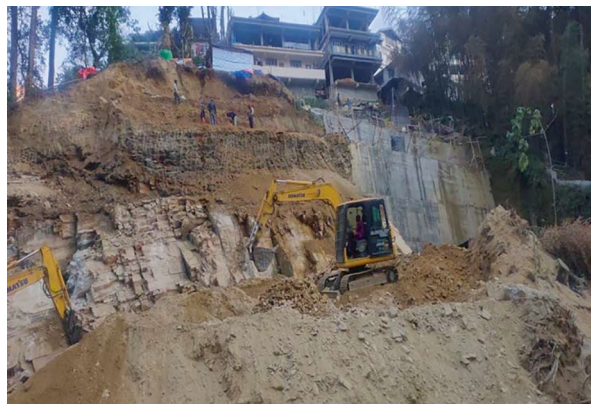
Plate 4 Slope instability due to construction activities at Gangtok, Sikkim (2.1.2024)
